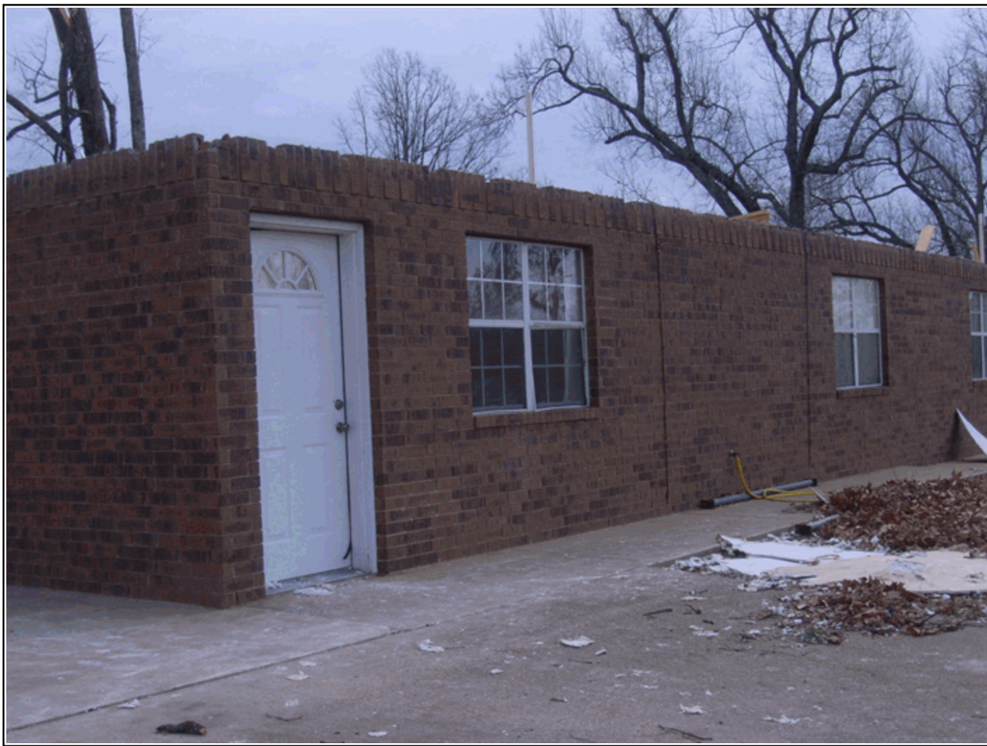
A severe thunderstorm tore the roof off a duplex during the early afternoon of December 9, 2012, between Gepp and Viola in Fulton County, AR. Photo by John Robinson, WCM, WFO Little Rock.
