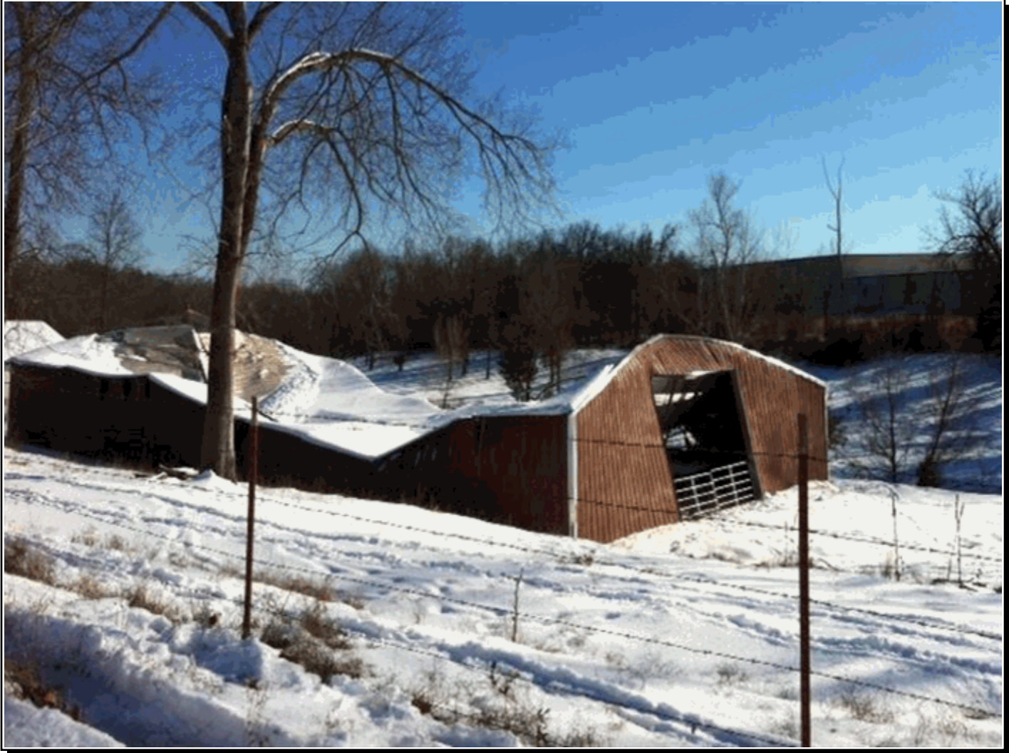
A barn being used as a storage building near Yellville in Marion County, Arkansas, collapsed from the weight of snow and sleet that fell on December 5-6, 2013. The photo is courtesy of Keith Edmonds, Marion County Office of Emergency Management.
