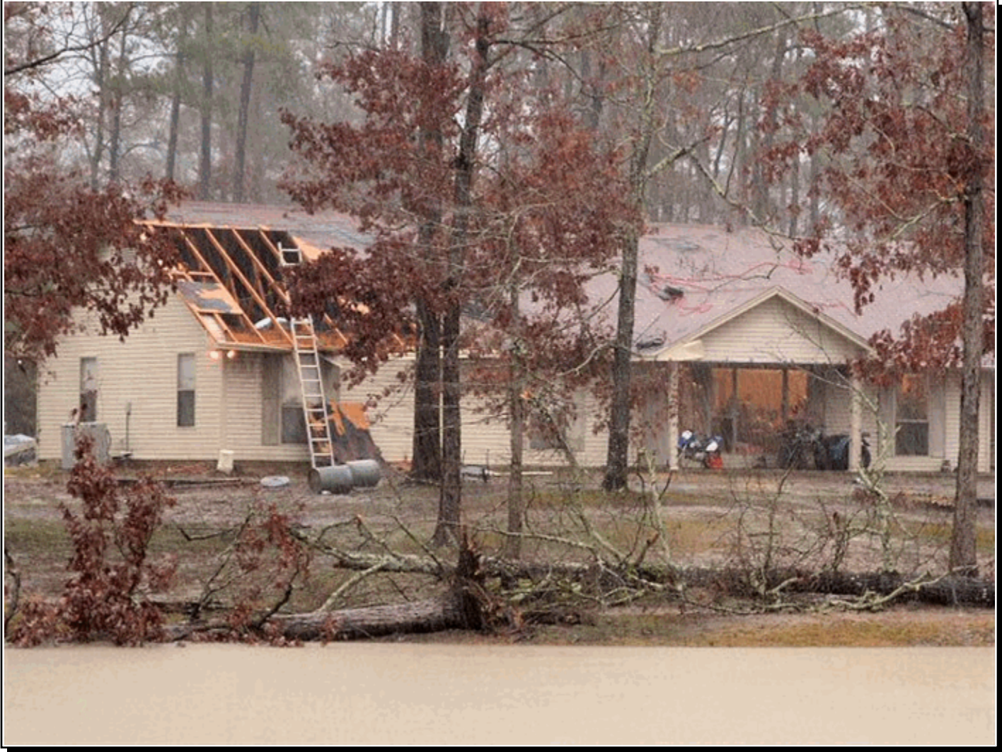
An EF1 tornado removed part of the roof of a house at Redfield in Jefferson County, Arkansas, on the evening of December 20, 2013. Photo by John Lewis, Senior Forecaster, WFO Little Rock.
