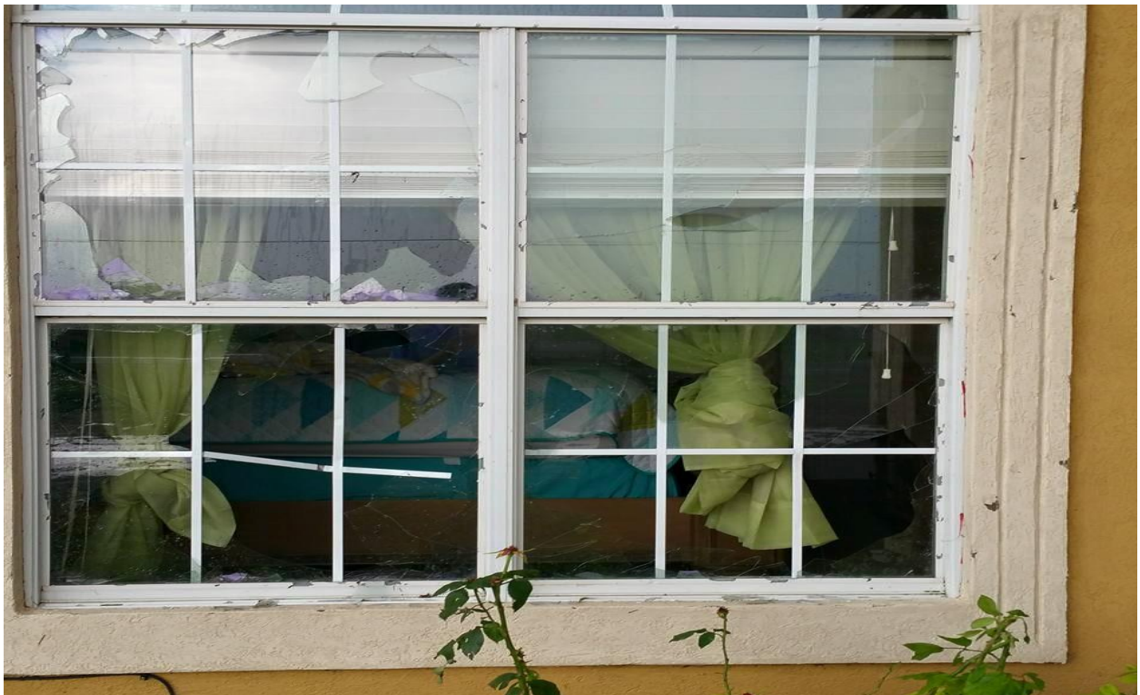
Figure 4 – Hail Damage to Residence in South Odessa (courtesy of CBS7/KOSA).
