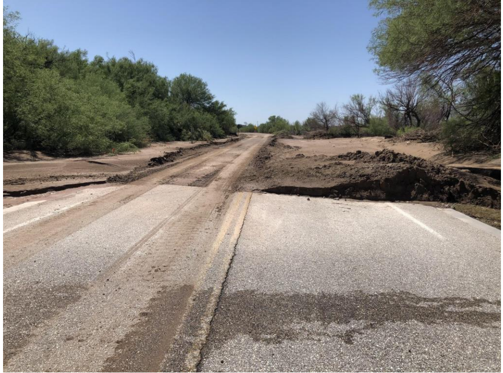
Figure 3: An area along Santa Elena Canyon Rd where a mud deposit had been cleared. Notice the area on the left where the mud hadn't been cleared yet; this mud deposit was several inches thick.
