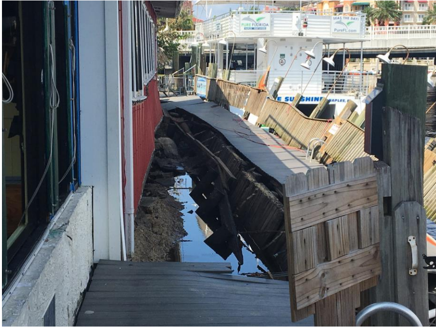
Damage to dock at Tin City in Naples caused by storm surge from Hurricane Irma (NWS Storm Survey picture)
