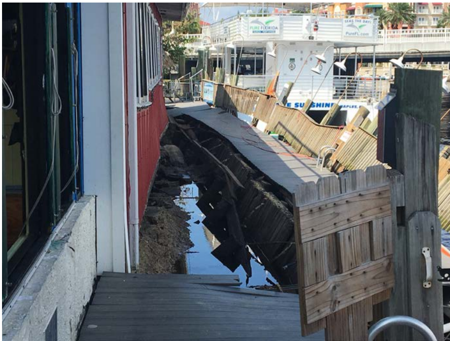
Damage to dock at Tin City in Naples caused by storm surge from Hurricane Irma (NWS Storm Survey picture)
