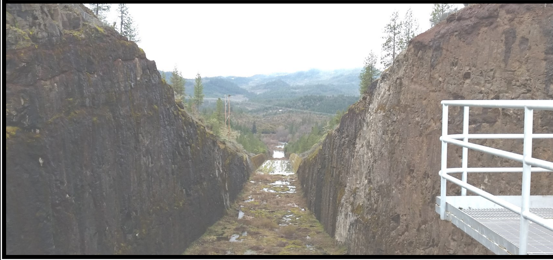
View of the spillway from above the spillway gates. Photo Credit: Misty Duncan, NWS Meteorologist
