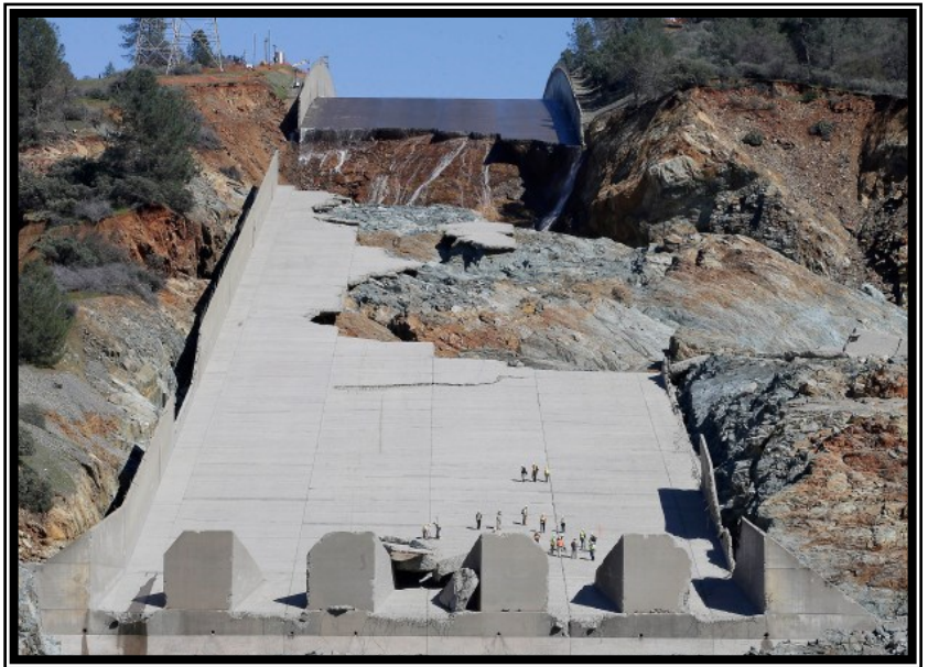
Oroville Dam Spillway with significant erosion damage on Feb 28th, 2017. Glancing at the workers on the spillway gives you a sense of the enormity of the situation. Photo credit: Mercury News
