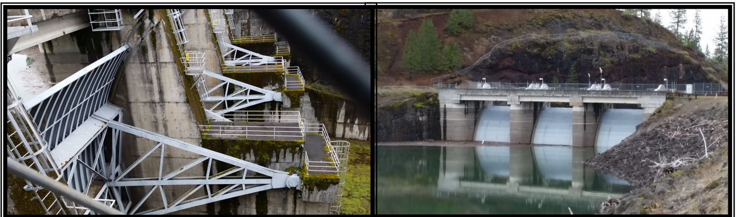
Spillway gates at Lost Creek Dam (Jackson County Oregon), from the lake side (right) and spillway side (left). Photo Credit: Misty Duncan, NWS Meteorologist
