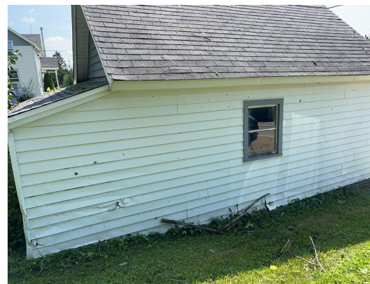
NWS MKX storm survey damage in Colgate, showing damage from debris flug up into an outbuilding.
