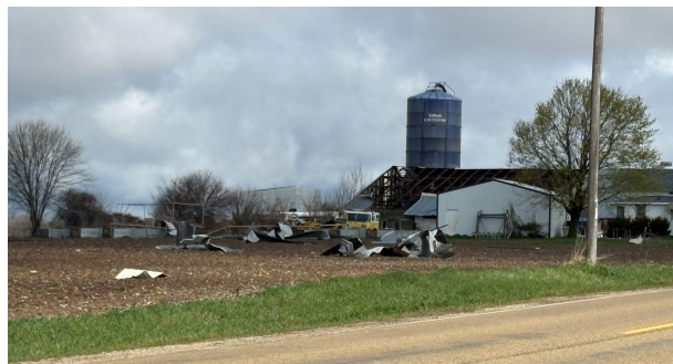
Barn damage near Elkhorn. Image courtesy of Brendan Johnson/TMJ4 Milwaukee
