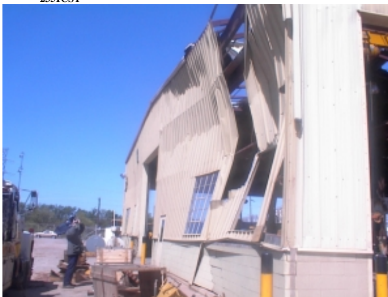
Tornado damage to a sheet metal building in downtown Wichita Falls.
