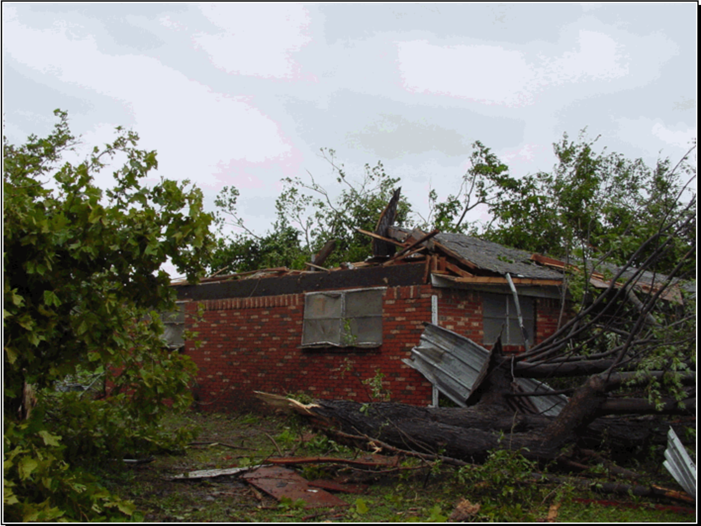
House Damage near Colbert, OK. Photo courtesy of Pete Covey.
