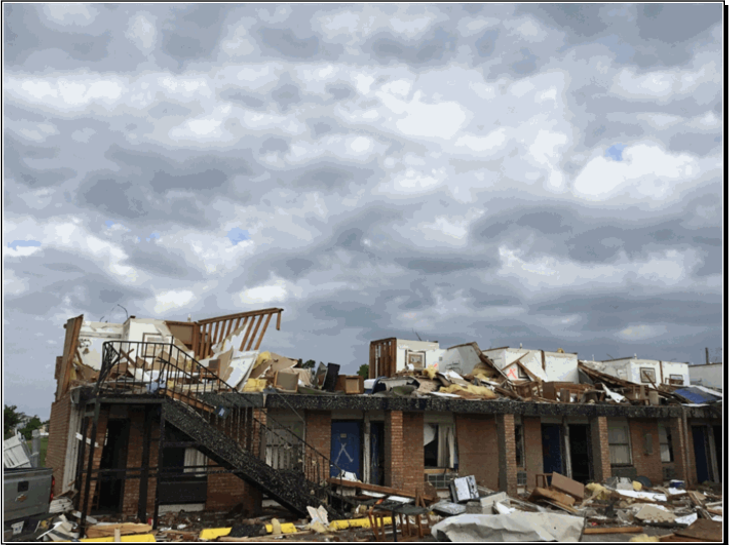
This motel on the south side of El Reno suffered significant damage from an EF3 tornado on the evening of May 25. Photo by Richard Smith, NWS Norman.
