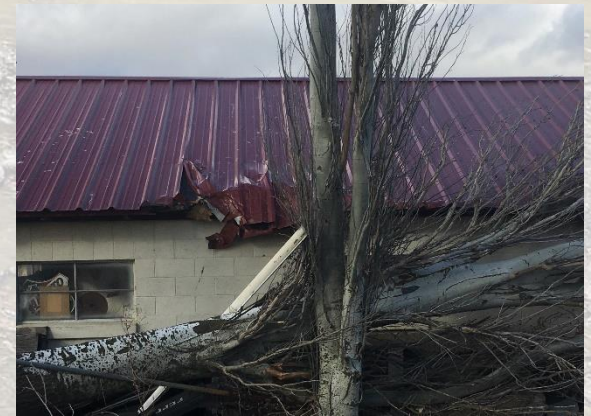
Thunderstorm wind damage in Grass Valley, OR. Photo by: Daniel Earl.
