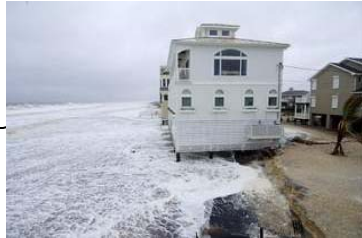
Water washes under homes Friday morning in Indian Beach, south of Dewey Beach. High tides caused beach erosion and flooding.
