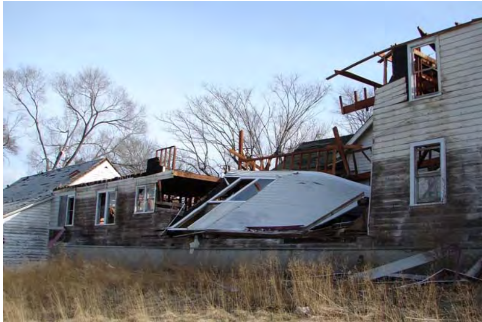
Two homes were damaged considerably by straight line winds in Knox County. In this photo, a connecting breezeway between the homes is shown.
