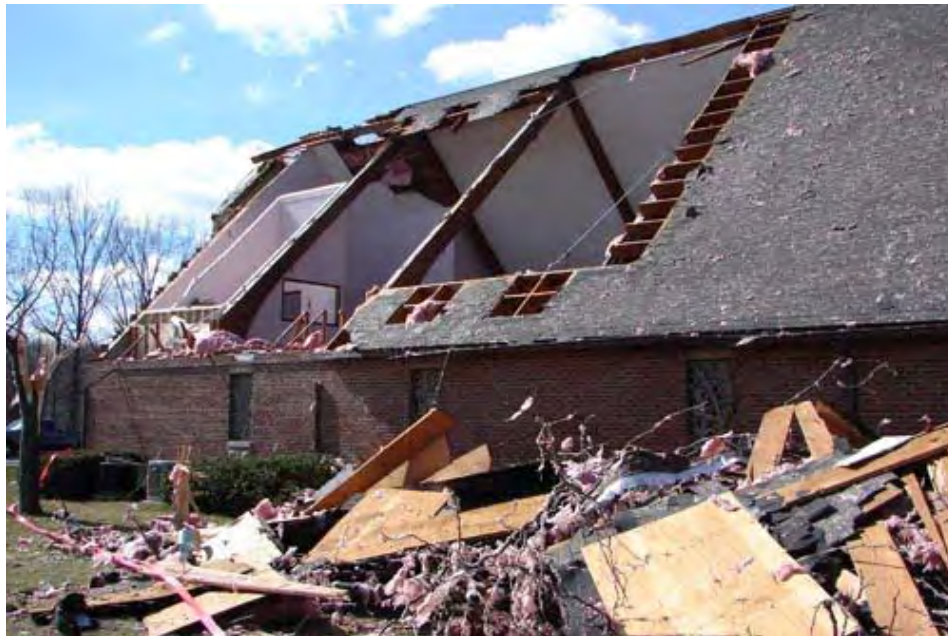
Part of the roof was removed from the Union Christian Church by a tornado on 16 February 2006. The steeple (not pictured), which had been atop the far end of the roof pictured, was found across the highway in a ditch after the tornado passed.
