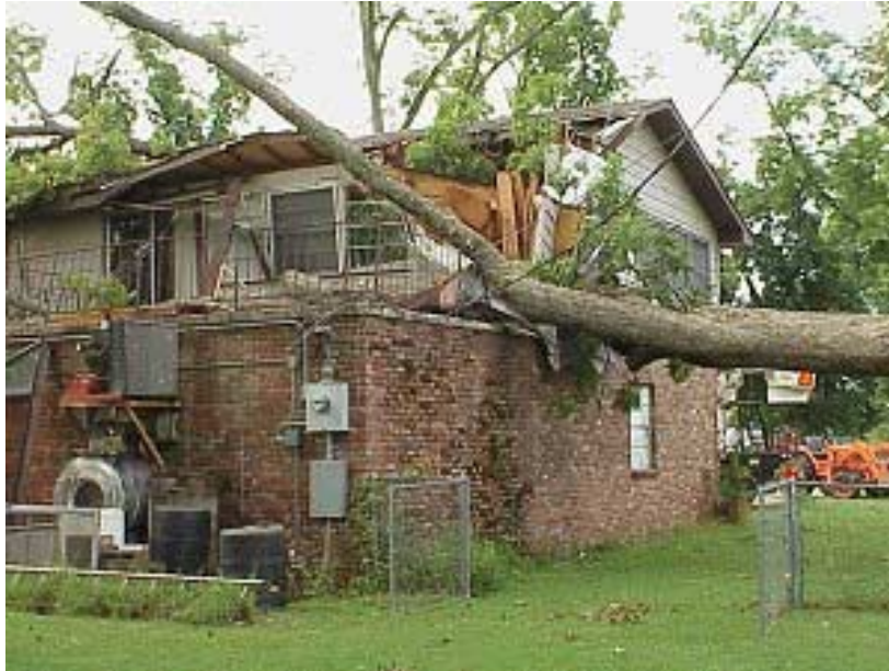
Damaging winds downed a tree onto a house near Scott (Pulaski County) around 11 pm CDT on 07/18/2002. Thunderstorm winds downed some large trees, one of which fell on a house. Numerous tree limbs were also taken down and a carport roof sustained damage.
