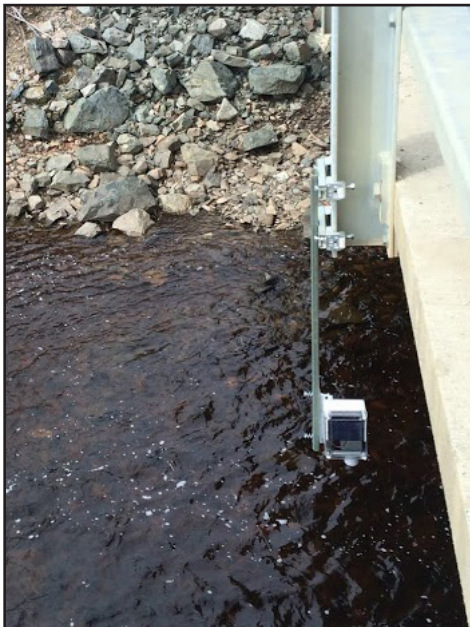
New iGage on bridge in Alaska.
