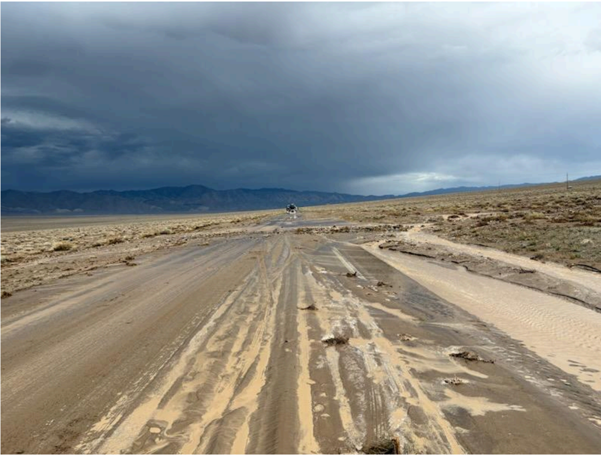
Photo 4. NV Hwy 95 near Luning closed due to flash flooding 8/13/26, image courtesy of NDOT
