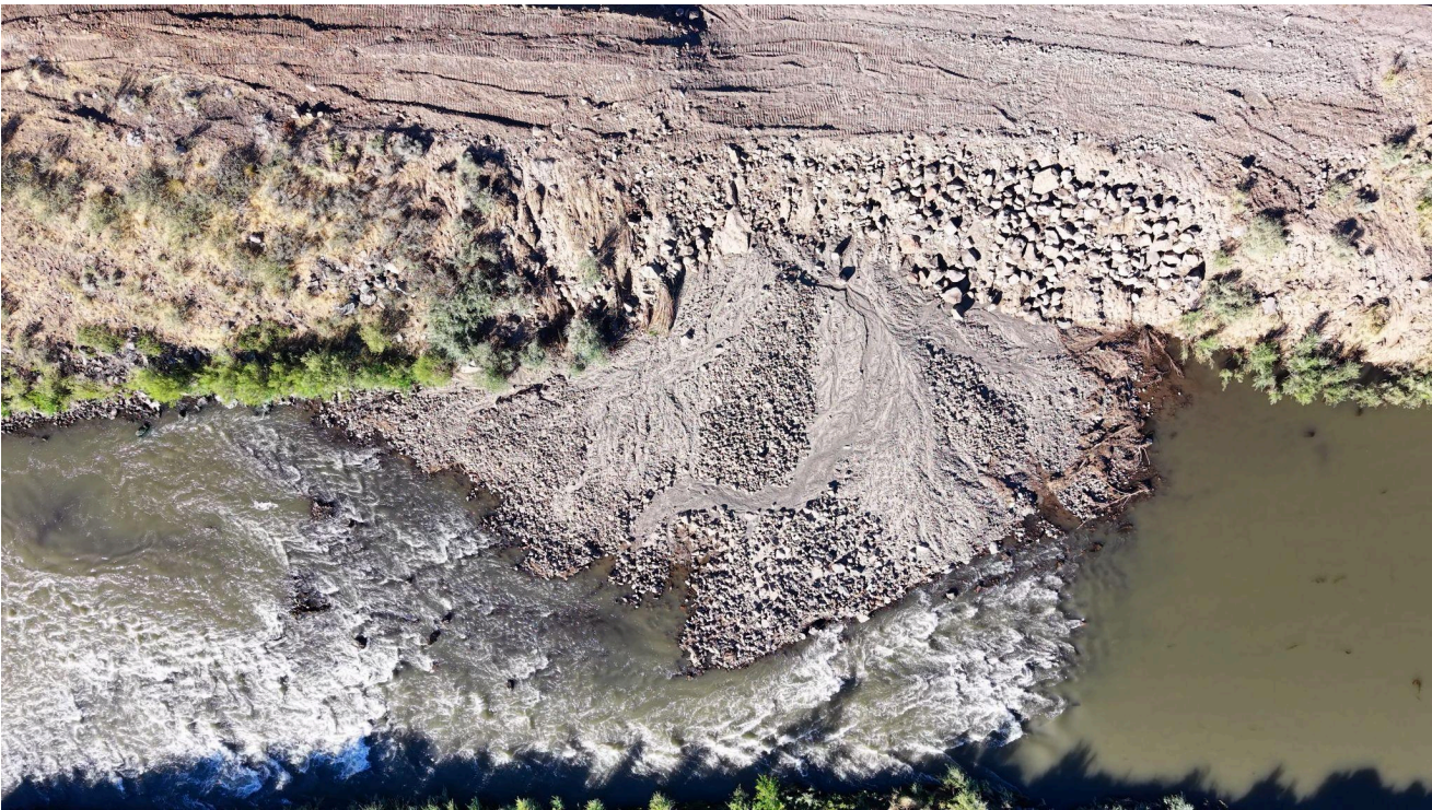
Photo 3. Debris flow partially blocking the Truckee River downstream of the Vista gage. Photo courtesy of Truckee Meadows Flood Management Authority.
