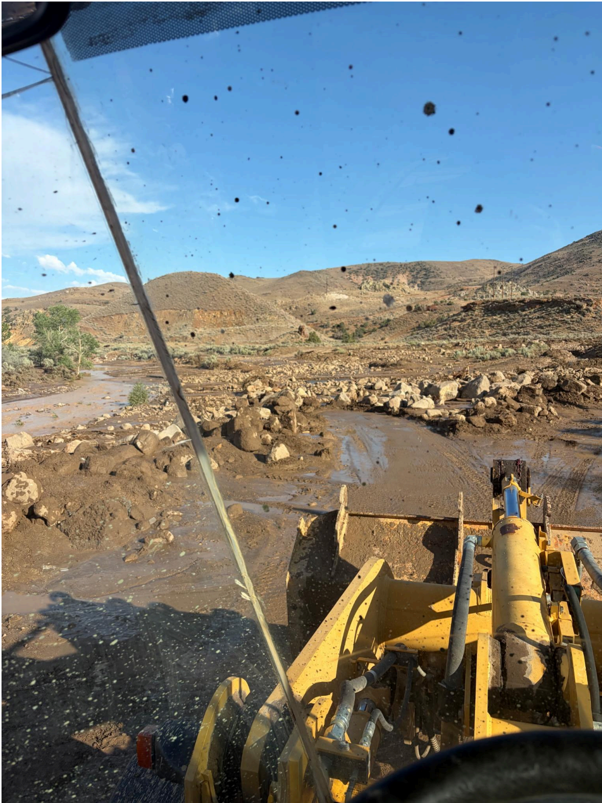
Photo 4: Clearing flood debris from Canyon Way along Long Valley Creek above Lockwood NV after the 6/19 flooding event. Photo courtesy of Storey County.
