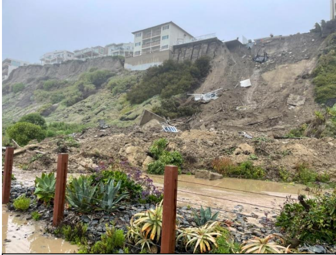
This hillside in San Clemente gave way on 15 March. There were no injuries, but it prompted evacuations (OCFA).
