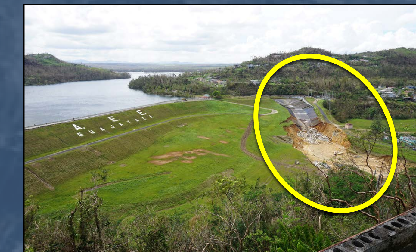
Guajataca Dam with compromised spillway.
