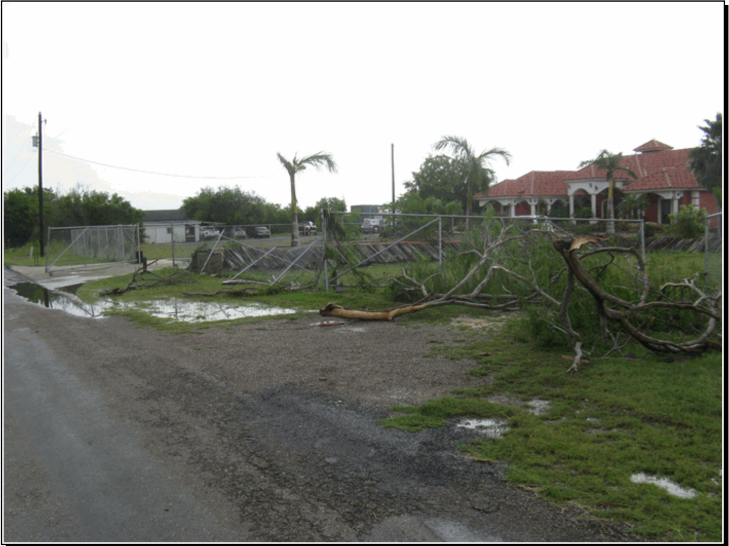
Damage to property and roof at a well built single family home in San Benito, TX from small tornado which contained estimated 80 mph winds. The large mesquite limbs were lifted from trees that could not be found on or near the property.
