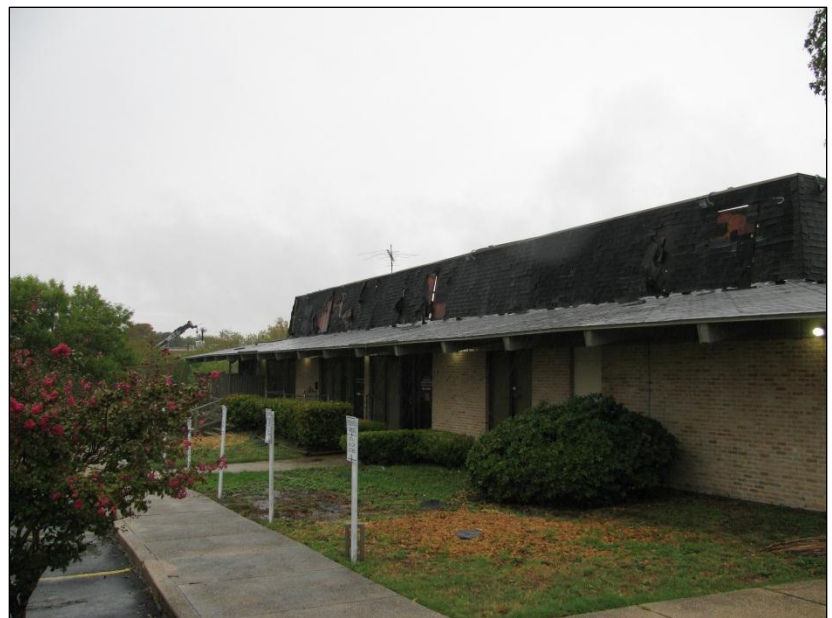
Roof damage at a business along Valley Hi Drive
