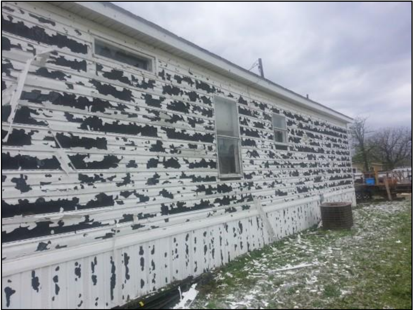
Figure 4. Hail damage to the side of a mobile home near Kingsland, TX, on April 2, 2013.
